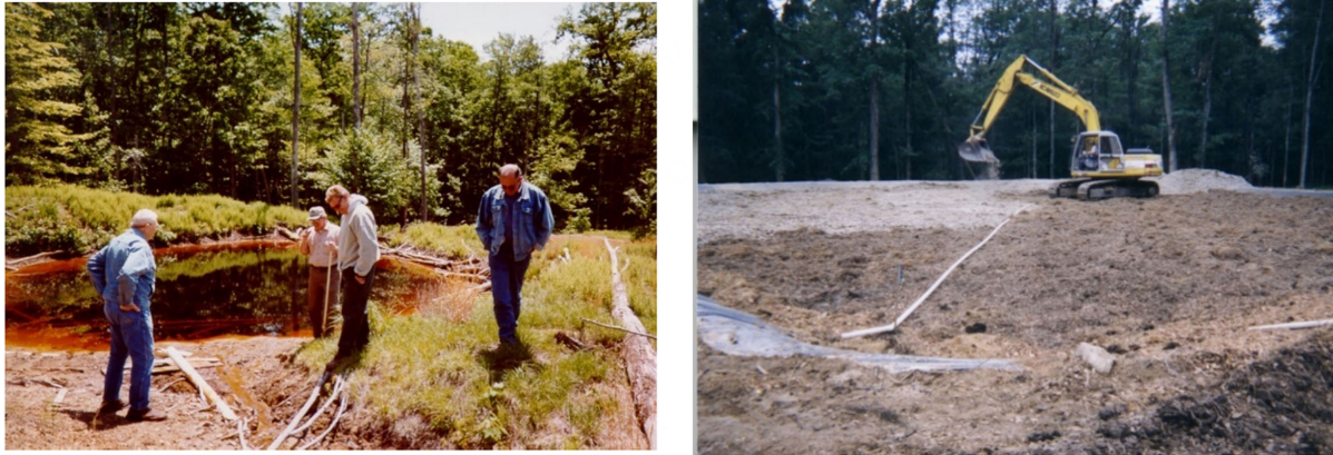
Figure 9. Fran Mine ARD and pilot BCR under construction prior to burial. BCR: Biochemical reactor; ARD: acid rock drainage.
