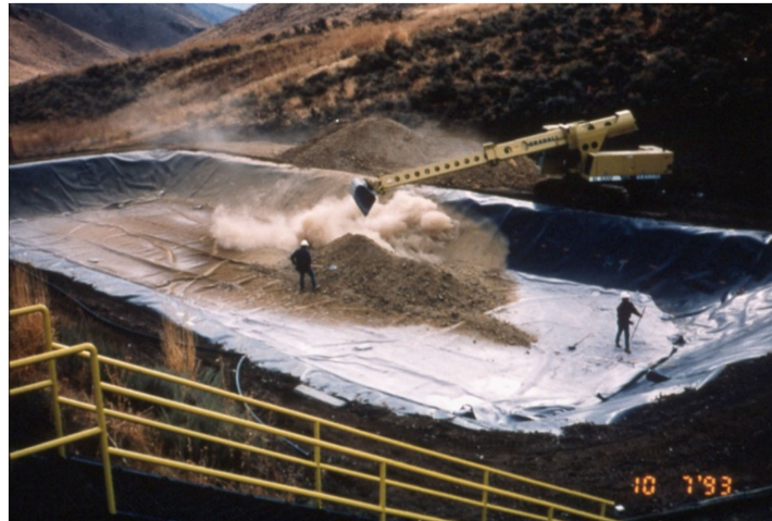
Figure 3. Dusty nature of BCR media evident in construction. BCR: Biochemical reactor.
